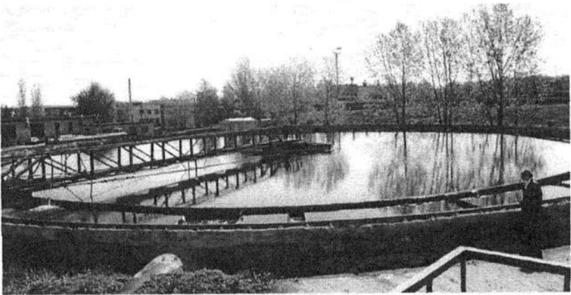
Figure 11. Clarifier used in a wastewater treatment plant.
